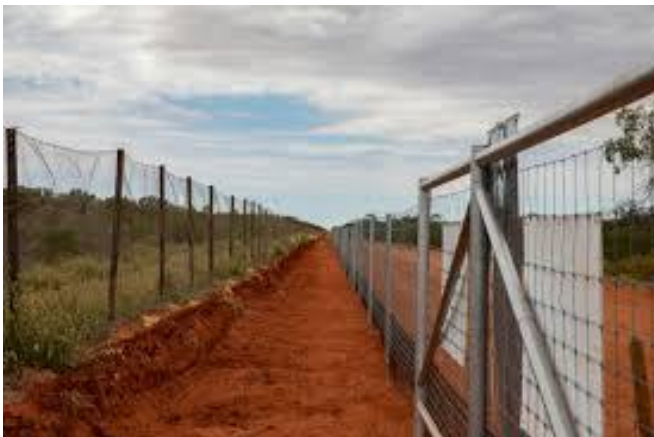
The Wild Dog Fence. This structure stretches across South Australia for 2,150 km from the Great Australian Bight near Fowlers Bay to the New South Wales border. More than two-thirds of the Dog Fence is being rebuilt in SA to protect our $4.3 billion livestock industry. (photograph courtesy of PIRSA)
